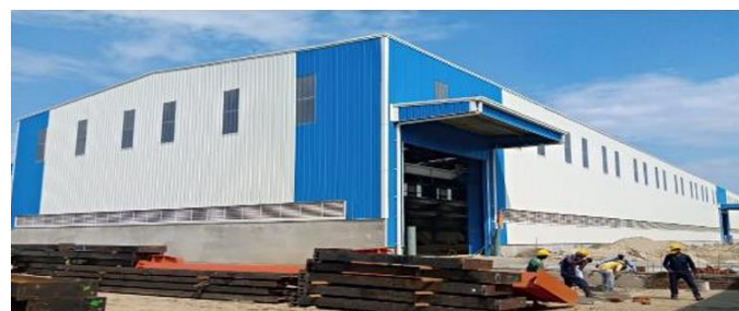
Tamil Nadu Manufacturing Facility I
