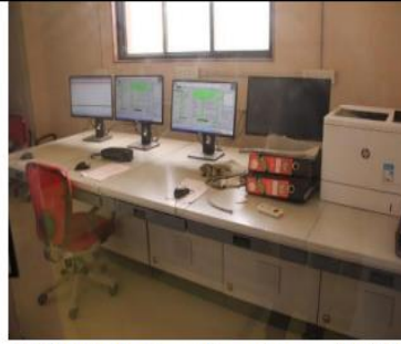
SCADA System Operations of EHV Substation
